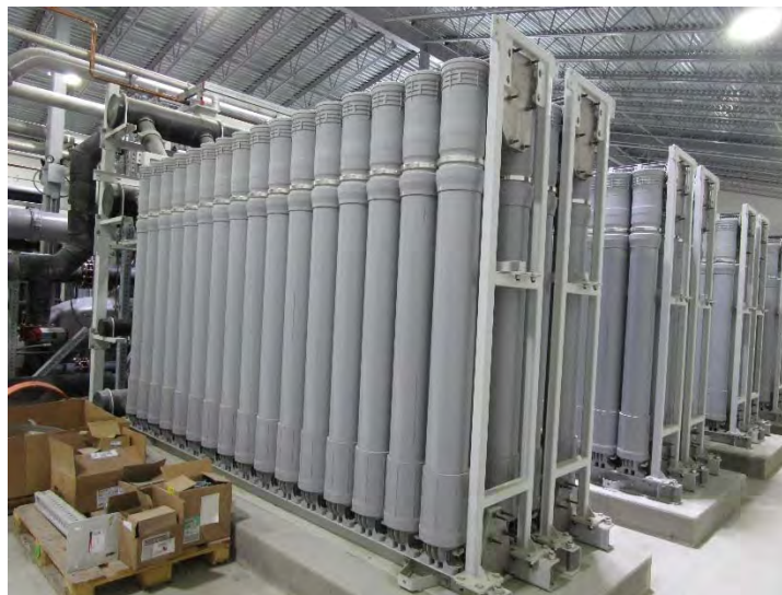
Figure 4-8. Photograph of ultrafiltration membrane skids
