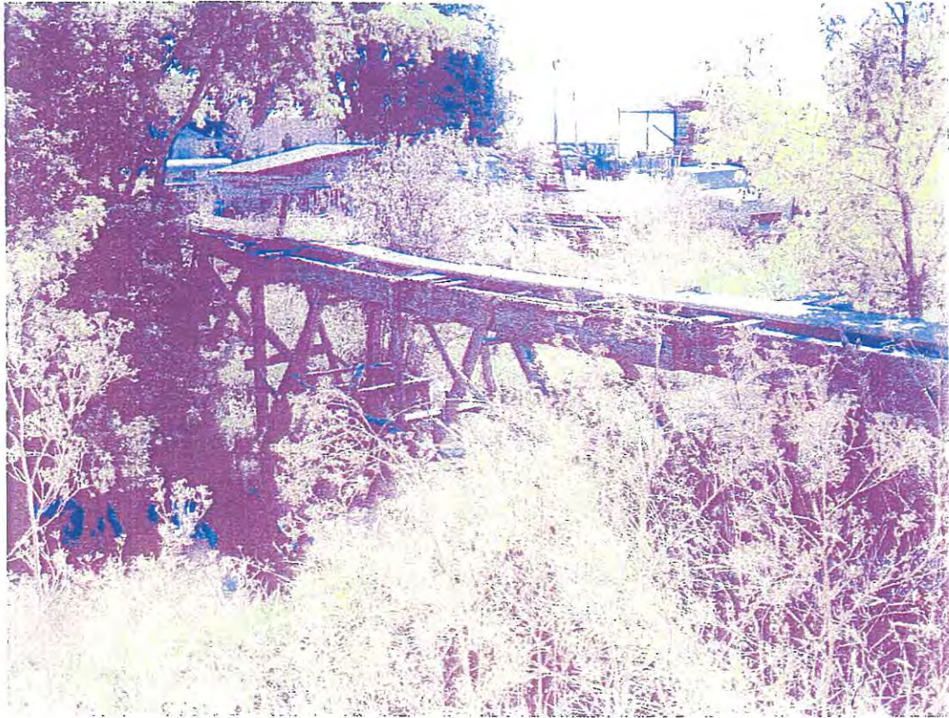
View of wooden aqueduct (M-2) looking southwest across Fivemile Creek and toward farmstead (M-3).
