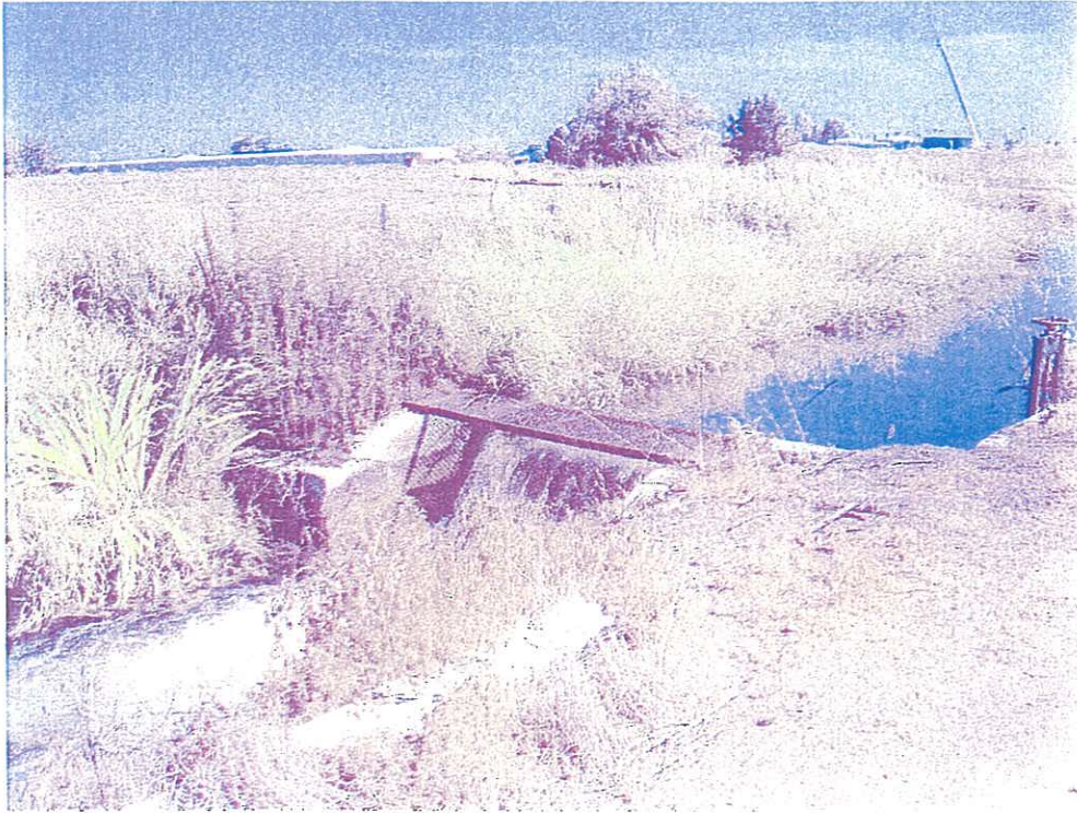
View of Creason Lateral looking southeast in NW ¼ of SE ¼ of Section 34.
